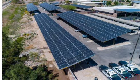
Solar Panels in the Policy Facility Parking Lot Source: SOLON Corporation
