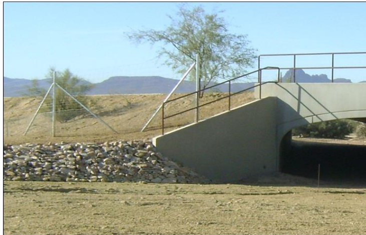
Figure 3. Example of wildlife fencing tied into culvert at Twin Peaks Road
